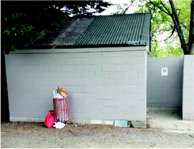
Figure 18: Public toilets and rubbish bin in East Gore.
